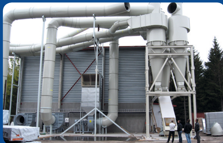
Airborne particles are removed from the air inside the building and ducted to the exterior for collection and disposal
